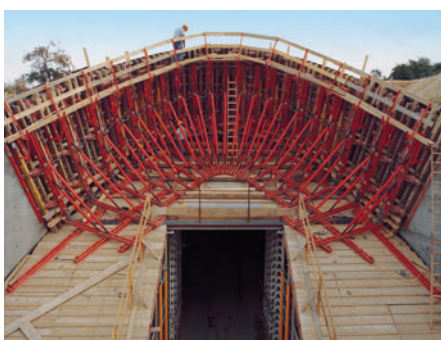
Elliptical-shaped tunnel portal with RUNDFLEX panels and accessories from the VARIO programme. The problem of constantly changing radii and inclination was solved by means of conically-cut filler timbers.
